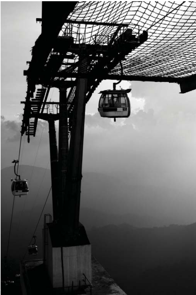
Figure 3. FORE system monitors cable car drive system.
